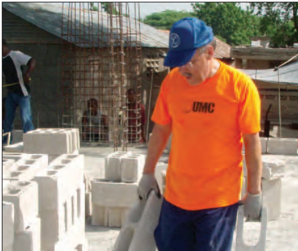
Gil Hanke carries cinder blocks to build the walls of the church at La Temblay, Haiti
